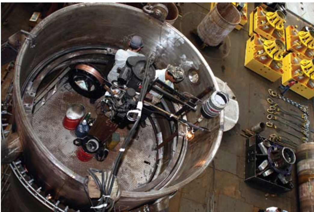
▼ Partial Production of shell of high-pressure reactor made in chromium molibdenium steel for HDT/HDS process.
