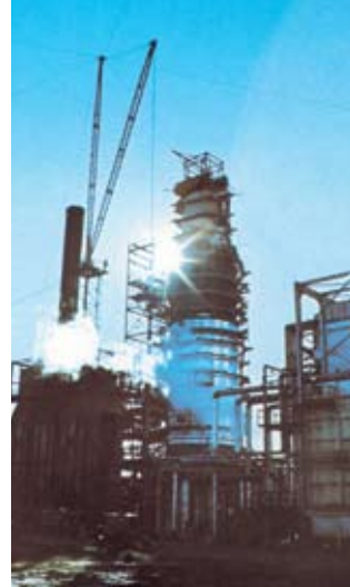
▲ Vacuum distillation column.
