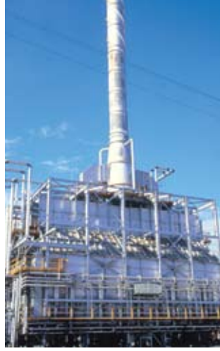
▲ Cabin-type fired heater.
