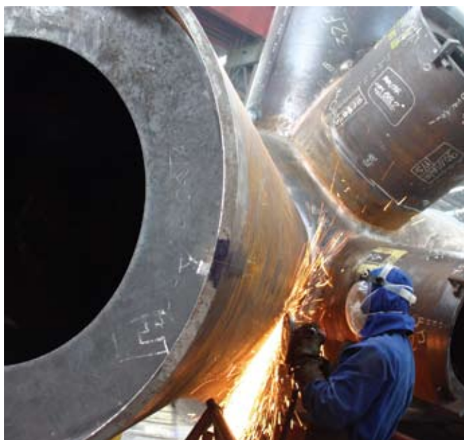
▼ Jacket for Fixed-Platform PRA-1, Petrobras.
